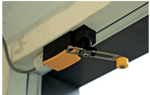
Insecure door contacts or roller switches that were costly to install were not considered for retrofitting the cabinet guarding system
